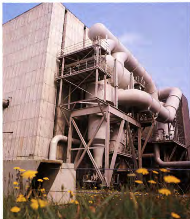
The in-house developed brine concentrator at Hengelo uses low-grade waste heat of approximately 50°C for concentrating brine to its saturation point. In view of the low waste vapor pressure, 3-m dia. piping must be used.
